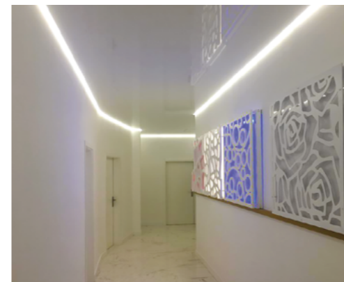
Health center Tenerife Spain / Tenerife Installer: Alemas
